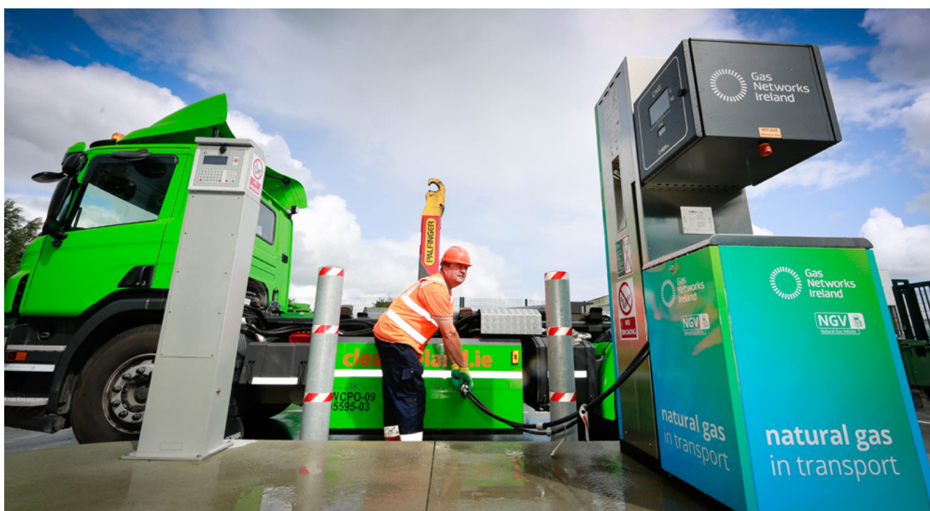
Figure 8-2: Clean Ireland Recycling Fast-fill CNG Station
