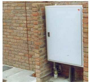
Six meter cabinet
