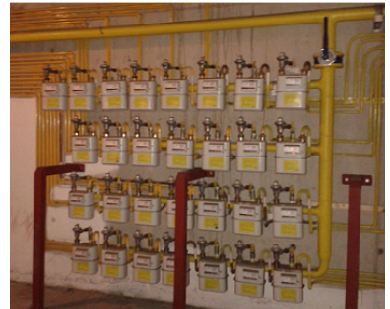
On-site meter manifold
