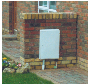
Domestic meter box
